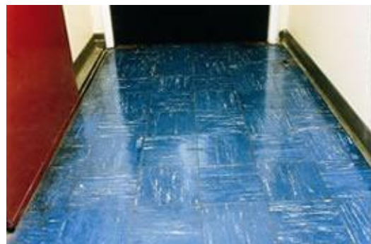
Asbestos containing floor tiles in a corridor
