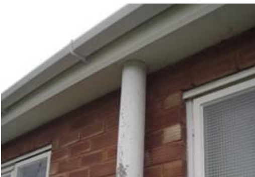
Asbestos cement drainage pipe (downpipe)
