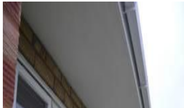
Pieces of Asbestos Insulating Board (AIB)
