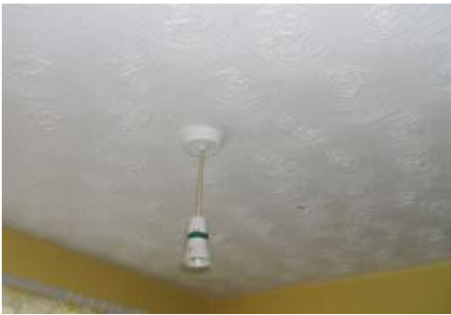
Asbestos textured coating
